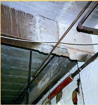
Sprayed Asbestos and Lagging.
